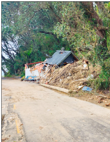
While Coastguard's Titirangi-based rescue vessel is at the OBC pending repair, its French Bay building, which suffered irreparable damage during the floods, has since been fully cleared from its site.
