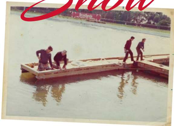
Volunteers build a temporary floating jetty in the pool at the Epsom showgrounds. (Rankin family pic)
